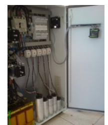
Three Phase Device
